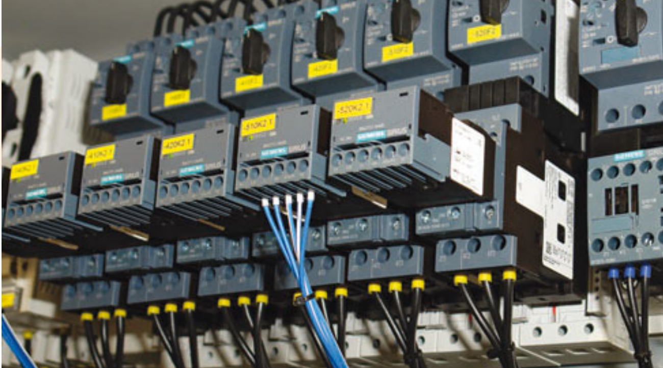
A tangled wiring mass with standardized Sirius connection components is a thing of the past
