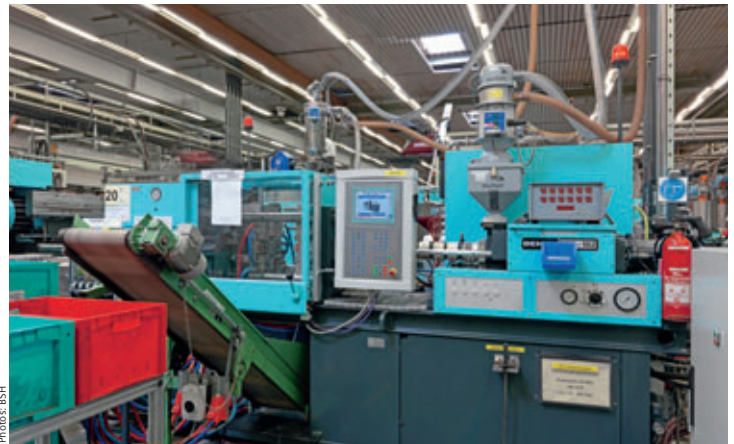
The retrofit allowed the electricity consumption of the Demag D60 NC3-P 600-182 to be reduced from 15 to 6 kilowatt-hours over an observation period of two weeks
