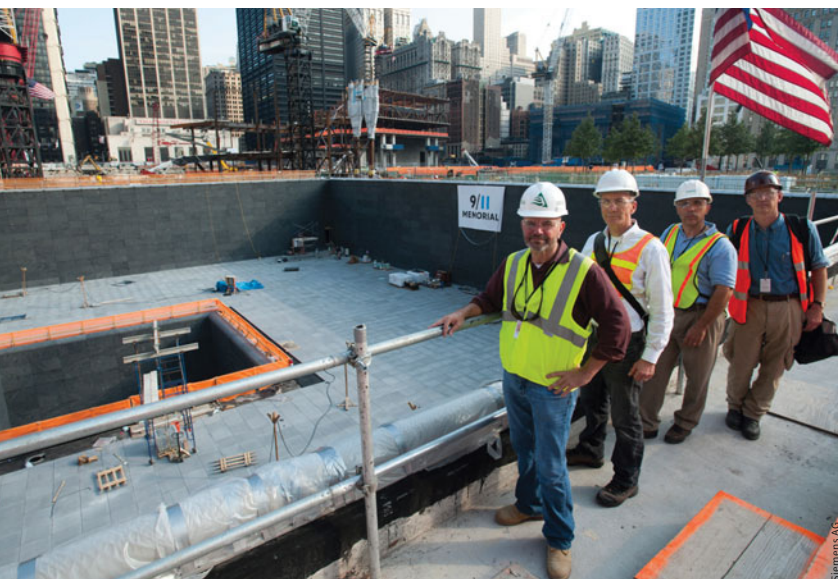
The memorial at Ground Zero required state-of-the-art technical solutions from the responsible engineers
