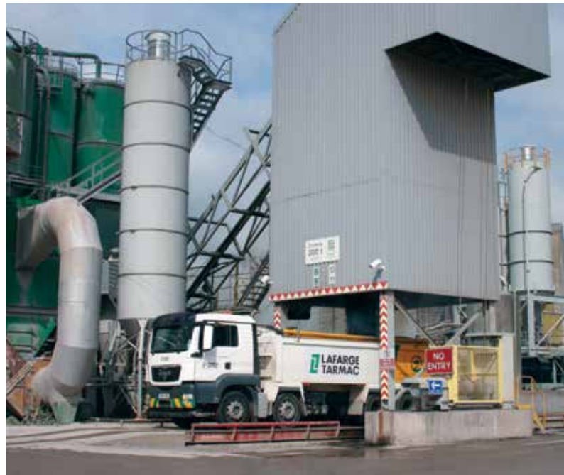
Trucks arrive daily to pick up hot asphalt from Lafarge Tarmac's finished asphalt storage silo. The SITRANS LR560 radar transmitter is installed at the top of the 10m narrow silo that houses the fibre.
