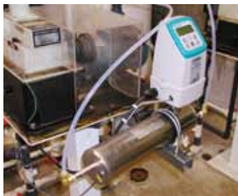
SITRANS FC MASSFLOW, MASS 2100 sensor with MASS 6000 transmitter, controls and doses the amount of polymers being used.
