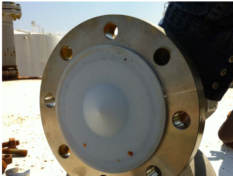
The corrosive and aggressive materials inside the process vessel did not affect the SITRANS LR250's performance in any way.
