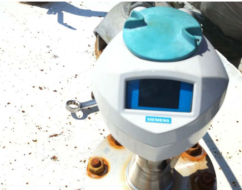
Installing the SITRANS LR250 was easy and the company now has reliable, high-performance continuous level measurements on their process vessel.
