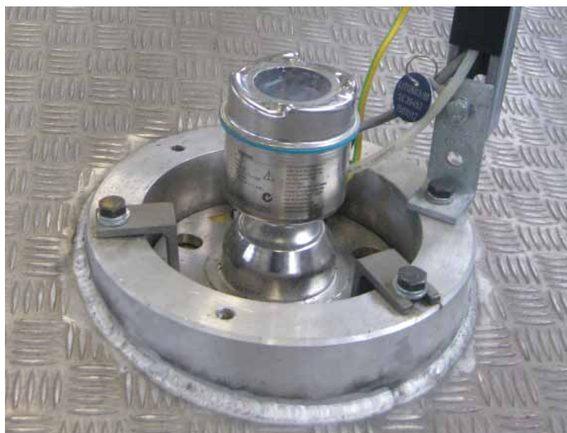
Operators easily installed SITRANS LR560 onto the filling silos and have seen a reduction in cleaning costs along with an increase in product quality.
