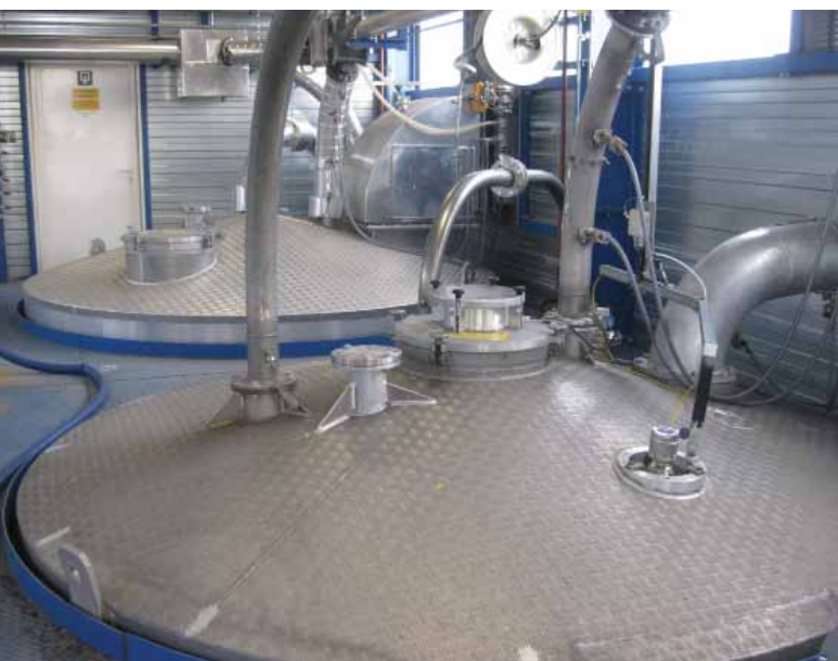
DSM Specialty Compounds rely on SITRANS LR560 for accurate and reliable level readings in this challenging application.
