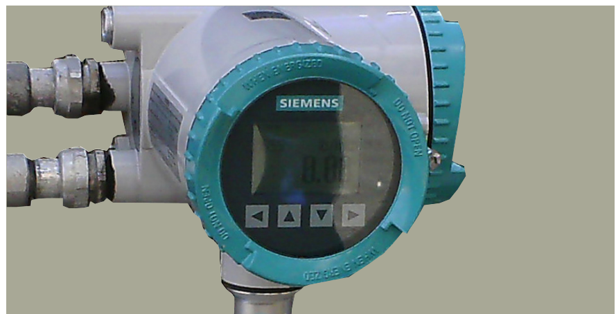
Siemens Coriolis transmitters monitor onsite flow operations and transfer flow, density and temperature data to the facility’s control system.
