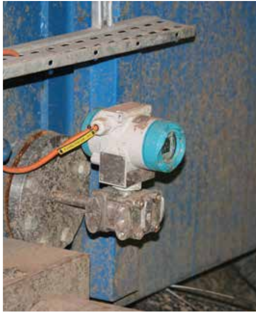
SITRANS P DS III measures liquid levels in ammonia removal tanks.
