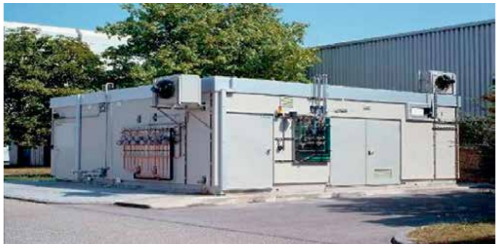
Fig. 13: Analyzer house (shelter)
