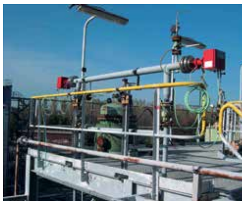
Fig. 5: Installation example of a LDS 6 in by-pass configuration to the main process gas stream
