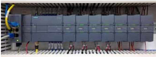
S7-1200 in mechanical room panel
