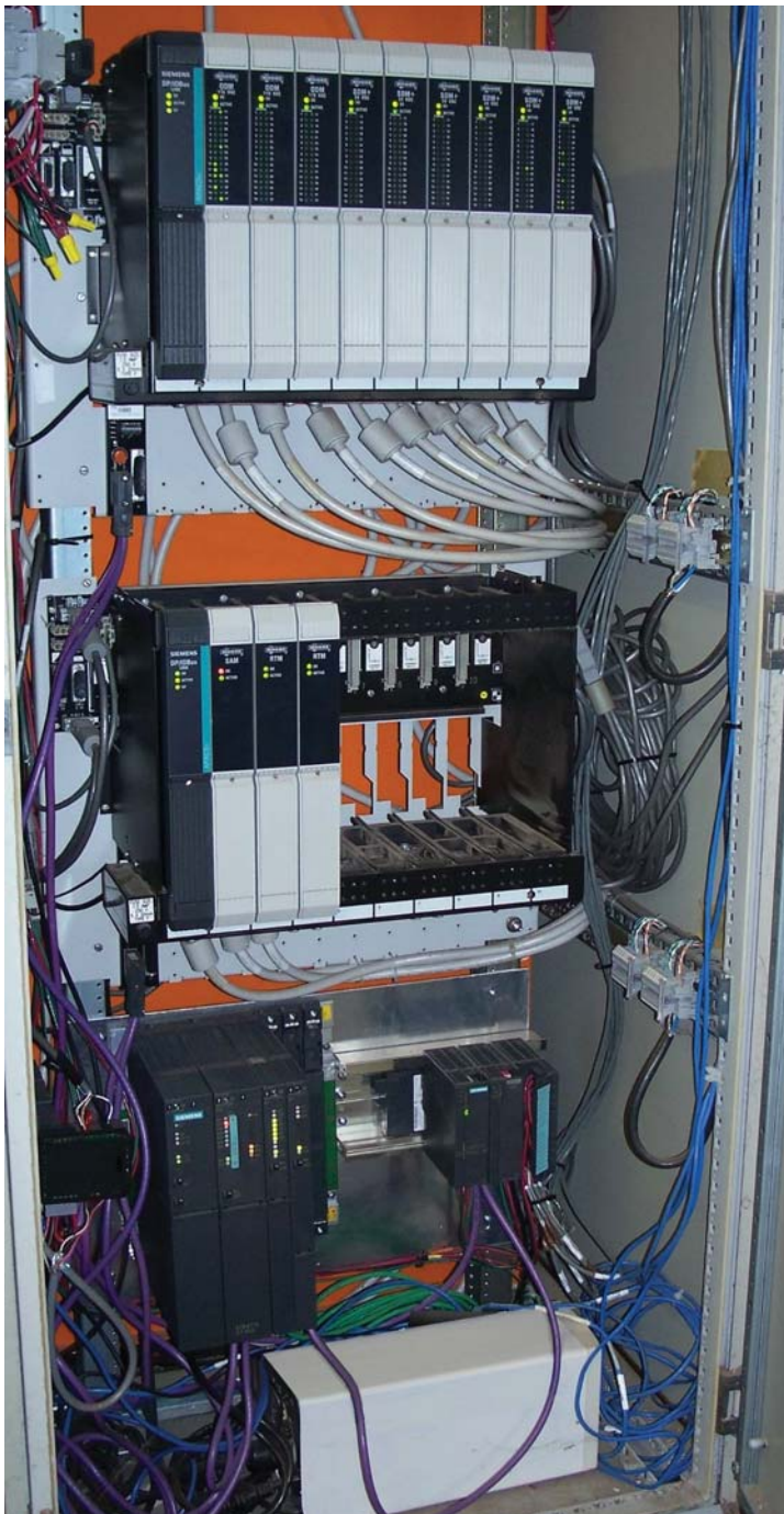
APACS+ I/O racks with DP/I/O Bus link modules connected to a PCS 7 controller installed at Four Roses
