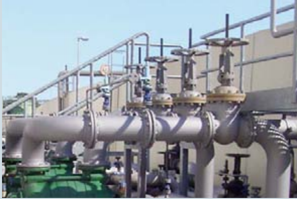
MICROMASTER inverter ensures cost-efficient diesel transportation at Shell
