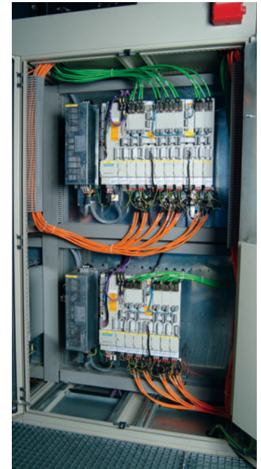
A Siemens SINUMERIK 840D with four CPUs occupies an electrical and HVAC control cabinet nearly 30' in length. Controls up to 60 axes and all auxiliary devices.
