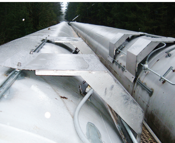
Custom covers protect the transducers
