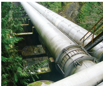
Penstocks running over a 150-foot deep gorge
