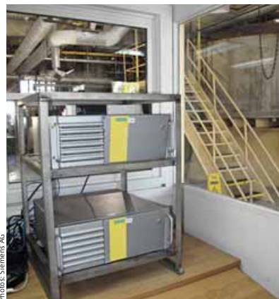
The new Simatic PCS 7 system has improved engineering and operation
