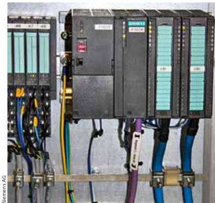
Siflow FC070 in the Simatic rack, fully integrated in the automation system via an ET 200M Profibus node
