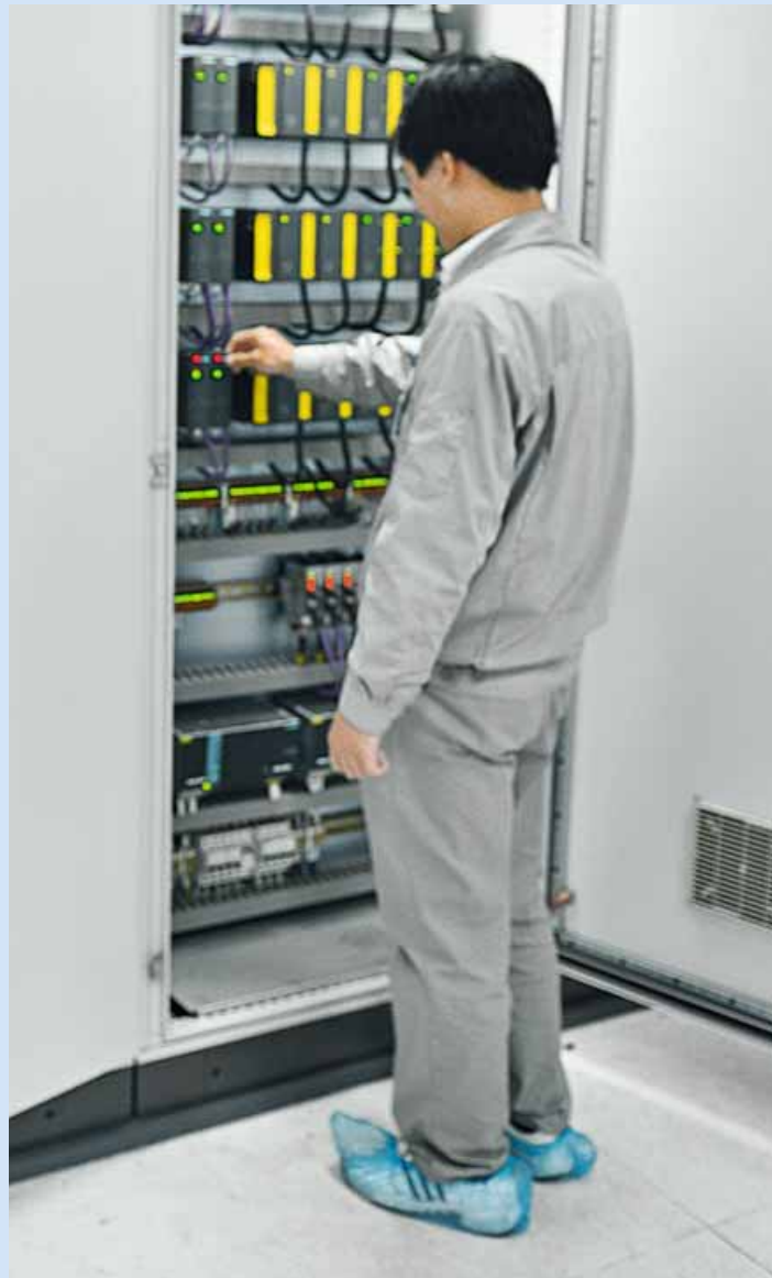
The integration of fail-safe and standard automation technology provided by Simatic PCS 7 supports increased reliability
