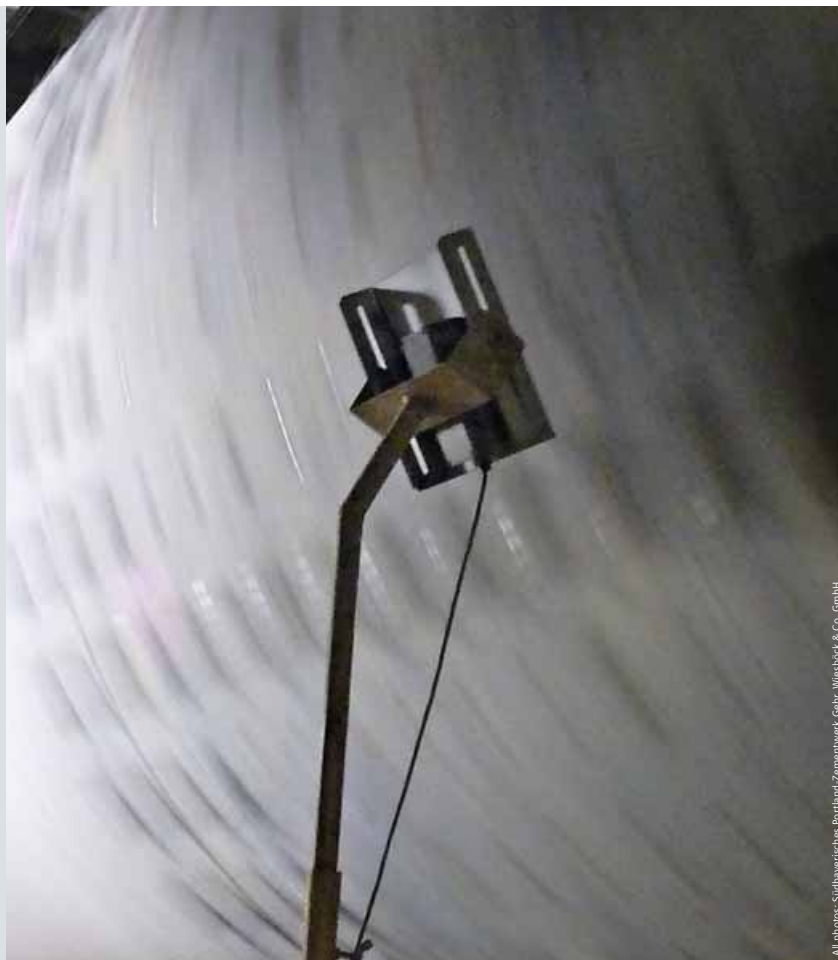
A sensor measures the filling level in the cement mill
