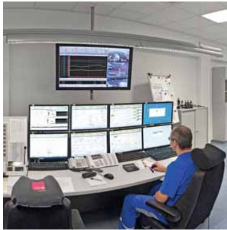
One of the first and largest remote operation centers uses a Simatic PCS 7 remote operation and control solution
